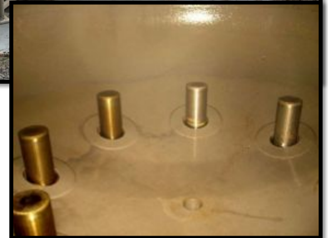
Right: Interior lining of GAC vessel with Septa underdrain design
